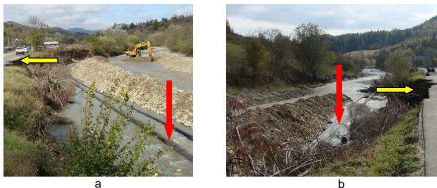
Fig. 3 The degradation of the oil transport pipelines in the Bolătău area after the flood in June 2016 on the Tazlăul Salat River: a - upward view of the pipeline position; b - downstream view (shoreline at DC180A with pipe stripping, photo oct 2016).
